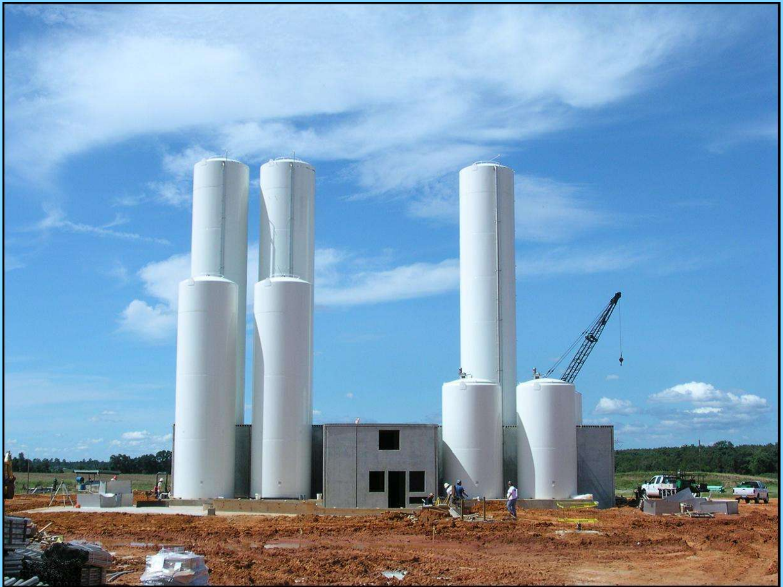
Ultra Filtration Plant – Baconton, Georgia
